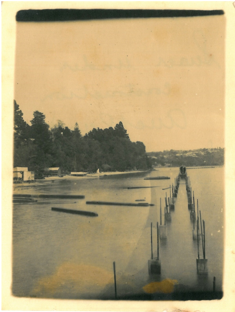
Figure 2: Photograph showing the main sewer line across Hobson Bay under construction, with Wilson's Beach to the left, c.1910-11. Note that there is no sign of the jetty at this time (Auckland Libraries Heritage Collections 1150-1).
